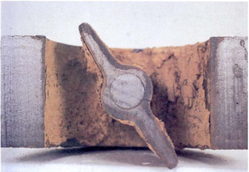
Fig. 31: Attack by graphitic corrosion in a water valve of cast-iron after 10 months' exposure to hot (50°C) sea water.
