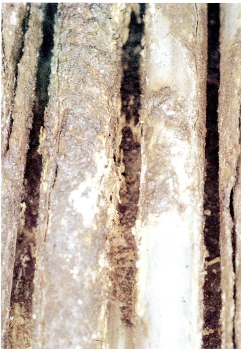
Fig. 127: Stress corrosion cracking in a bellows expansion joint of stainless steel for a district heating line; the attack has been caused by chloride-containing water dripping from the ceiling and evaporating on the hot surface of the bellows.
