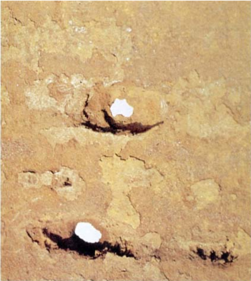
Fig. 23: Pits in oil tank of steel.
