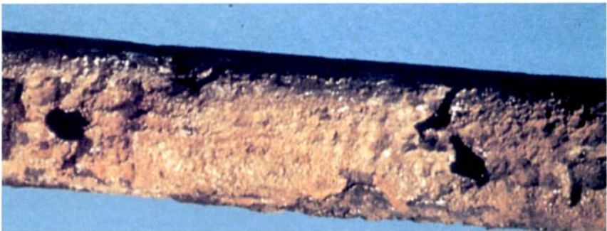
Fig. 29: Outside corrosion of a central heating pipe of steel located in a floor structure with damp mineral wool insulation; corrosion is caused by aeration cells at the beam: A, schematic overview; B, attack on the steel pipe.
